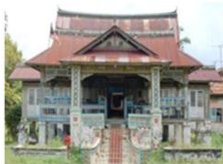
Figure-2. Condition of the house before the conservation work done.
