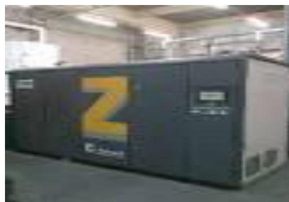
Figure-2. Water cooler compressor.
