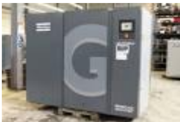
Figure-1. Air cooler compressor.
