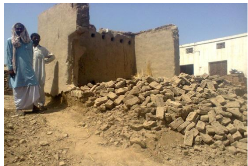
Plate- 2. A Damaged Mud Brick Room
