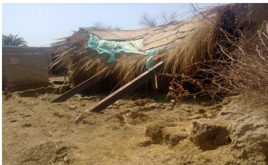
Plate- 1. A Collapsed Roof in Study Area
