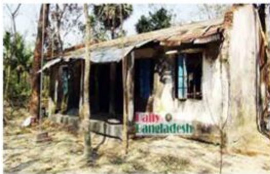
A rural school in a dilapidated condition
